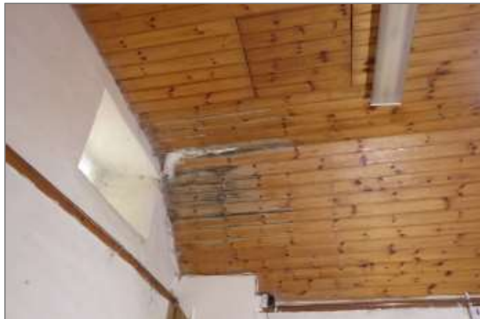
Miller's house: water ingress at roof level causing damage and fungal growth
