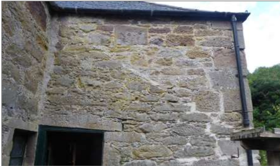
Meal mill: west elevation of the southern extension showing mortar repair patching at internal corner, open joints to the quoins, and settlement of the stone door lintol.
