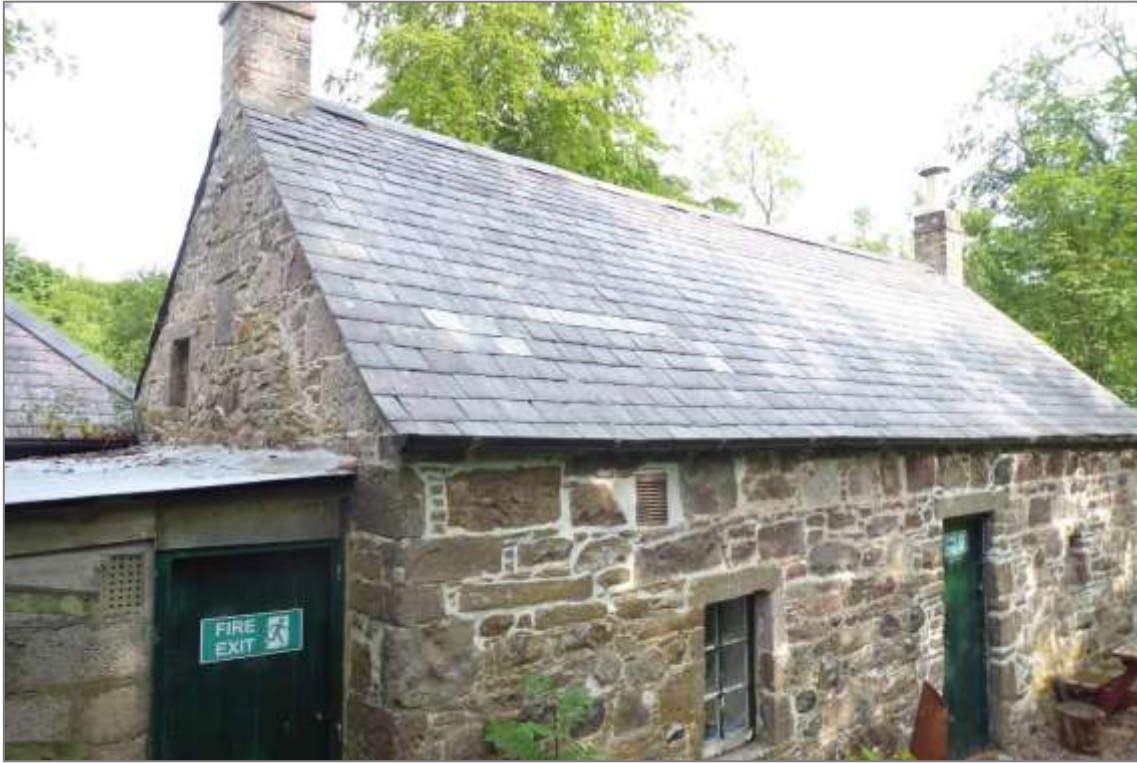
Mill of Benholm, miller's house rear elevation in 2023. Note the protruding masonry on the north gable suggesting an earlier wall with later build up supporting a raised or reconstructed wallhead for a later roof.
