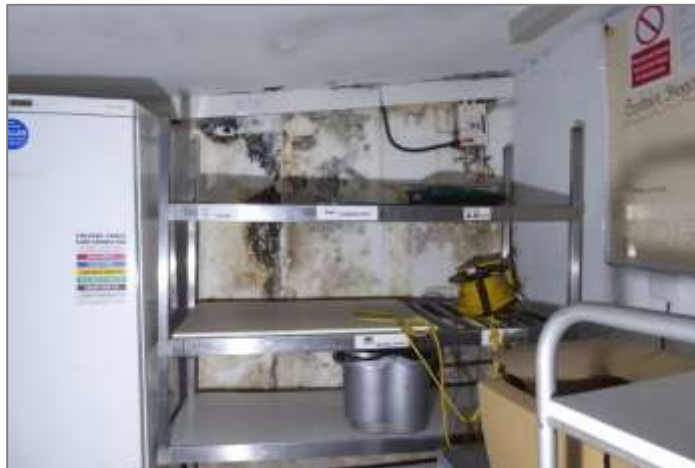
Below this gutter in the kitchen extension this wall is damp and covered in mould, including adjacent to the electrical distribution board.
