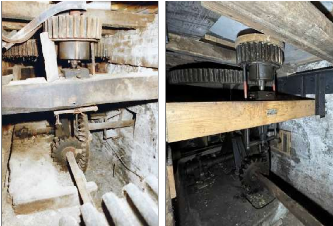
View of the primary machinery before restoration (left; WE Ltd image c1990-91) and in 2023 with the new bridge tree in the foreground and steelwork added to support the gearing structure and floor joists above.
