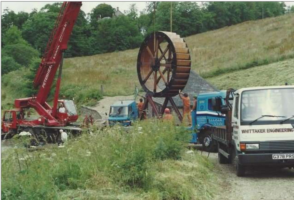
Whittaker Engineering Ltd installing the new waterwheel in April 1992. (WE Ltd image)
