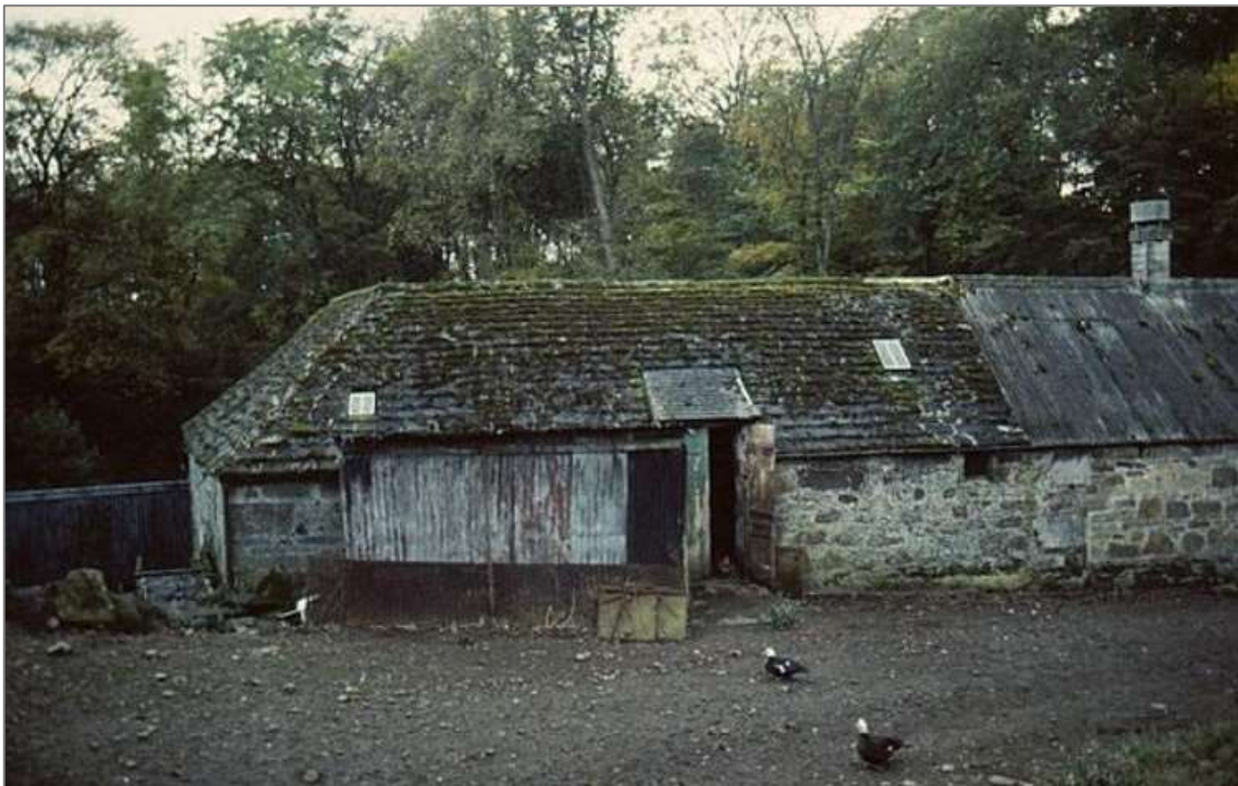
View of the Mill of Benholm in 1983 prior to adaptation showing an extension on the north elevation carried out in more 'temporary' corrugated iron sheet. Note the asbestos sheet roofing used to repair the kiln roof after a fire in 1971, and also the kiln vent (or piggy) of the same date. © Mills Archive Trust: JWN collection image 10751 https://catalogue.millsarchive.org/benholm2
