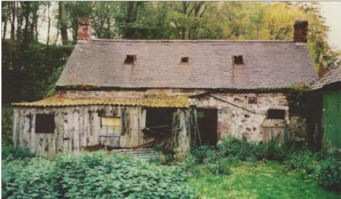
Mill of Benholm, miller's house in around 1986 awaiting repair and adaptation, note the timber and corrugated sheet extension probably added sometime from 1901 - 1923 (W&D DC postcard, © Aberdeenshire Council).
