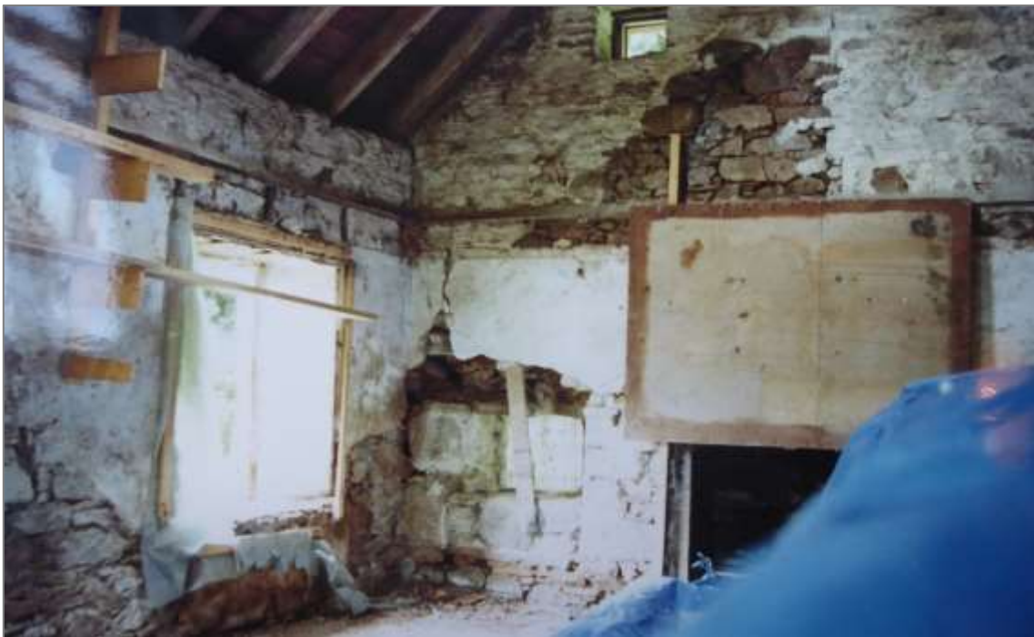
Mill of Benholm, miller's house in around 1992. The attic floor has been removed. The stripped back interior shows evidence of a possibly lower roof line showing as an unpainted part of the gable (HES file image).
