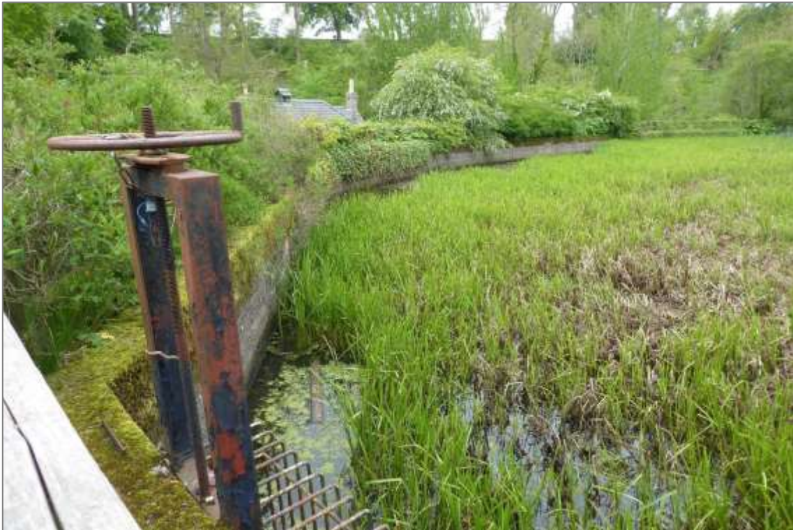
View of the mill pond in early summer 2023, note the low water level exposing the concrete retaining wall and rusting sluice. The pond is heavily overgrown with vegetation.
