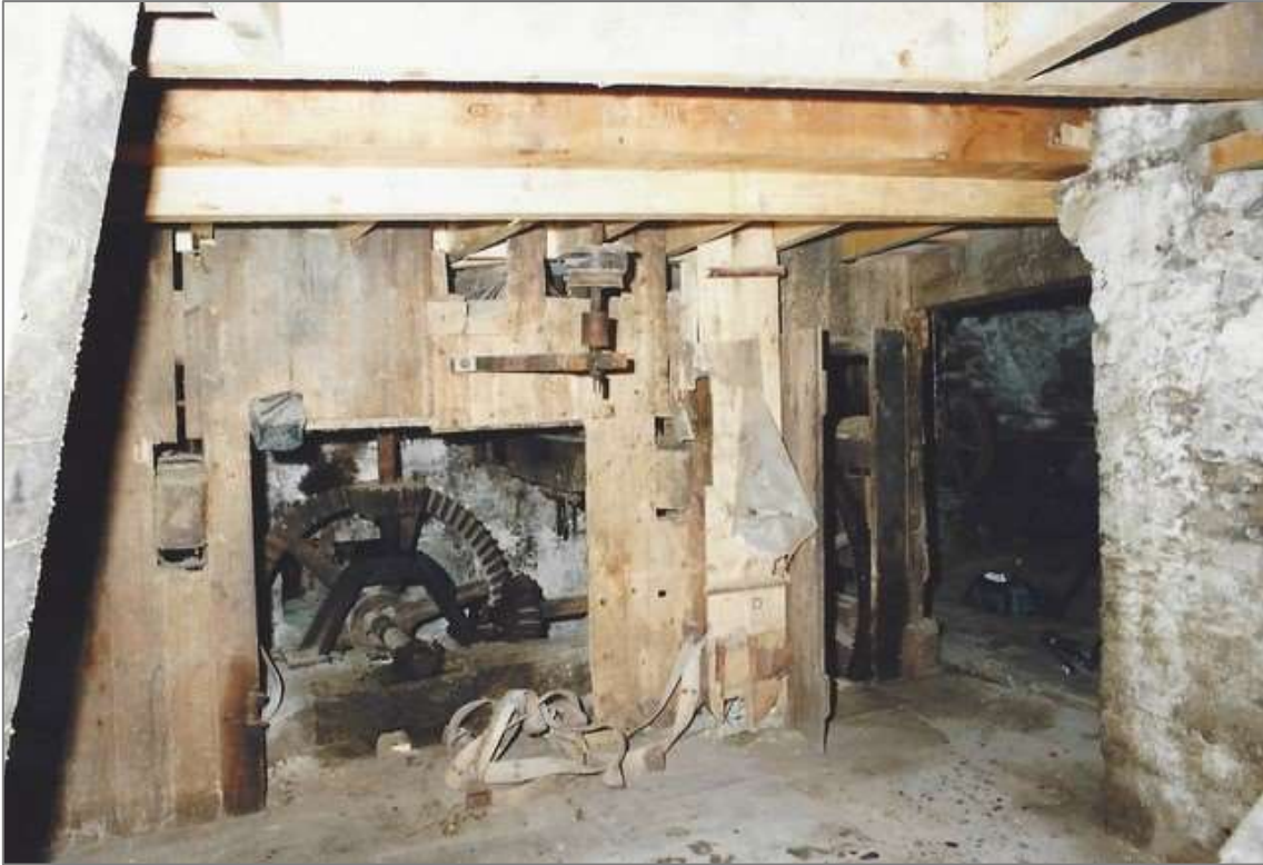
View of the gearing cupboard during dismantling for restoration, note the Meal Sieve & Small Fanner have been removed with a section of the timber walling but the form of the cupboard is largely intact including doors on the right. The Pit Wheel is visible inside. (WE Ltd image c.1990-91)
