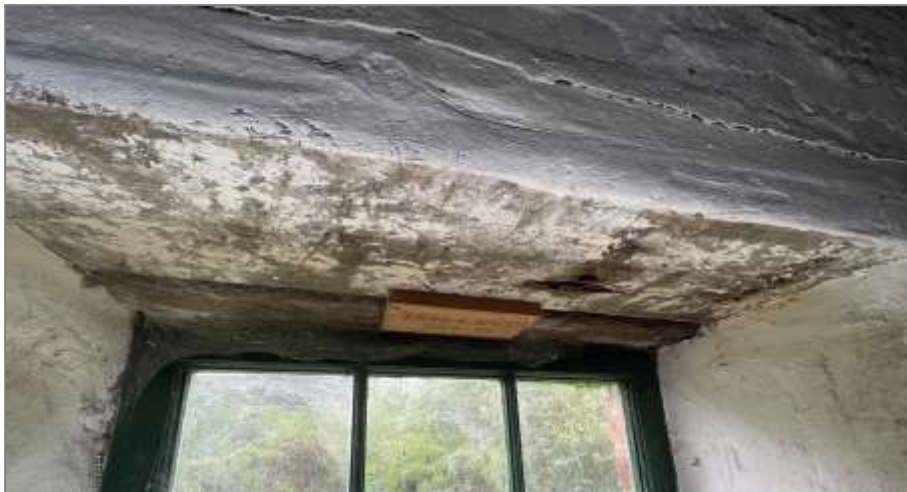
Meal mill: historic timber lintol over the 12-pane window on south elevation.
