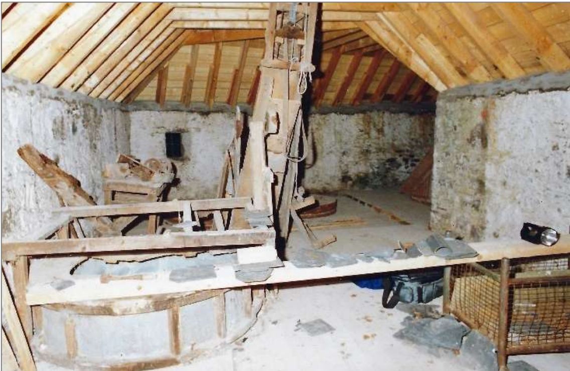
View of the meal mill interior during adaptation, note the cement based wallheads repairs (WE Ltd files).
