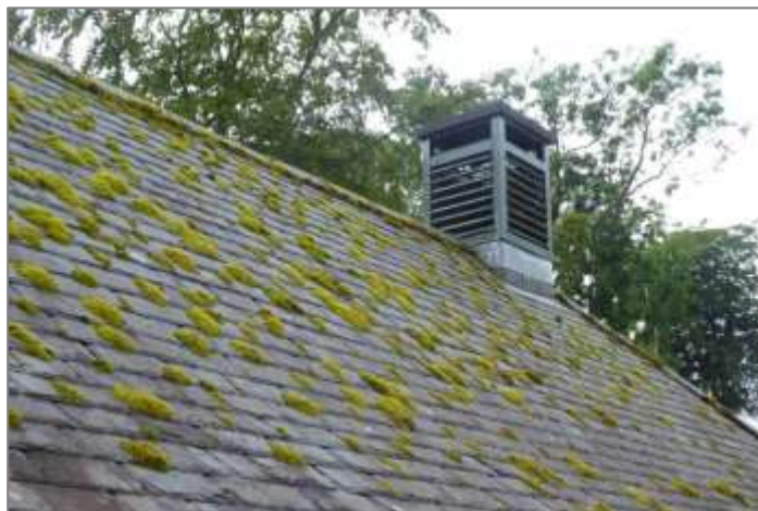
Meal mill: north roof pitch has a heavy moss build up. Note the inappropriate design of the current ventilator.
