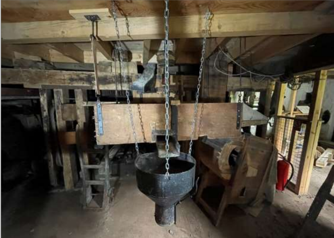
View of the gearing cupboard in 2023, note the restored Meal Sieve & Small Fanner back in place, however much of the timber walling which formed the gear cupboard has been lost.
