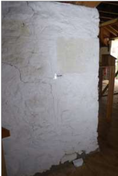
Meal mill: diagonal separation cracking where the earlier mill building wall meets the southern extension walls
