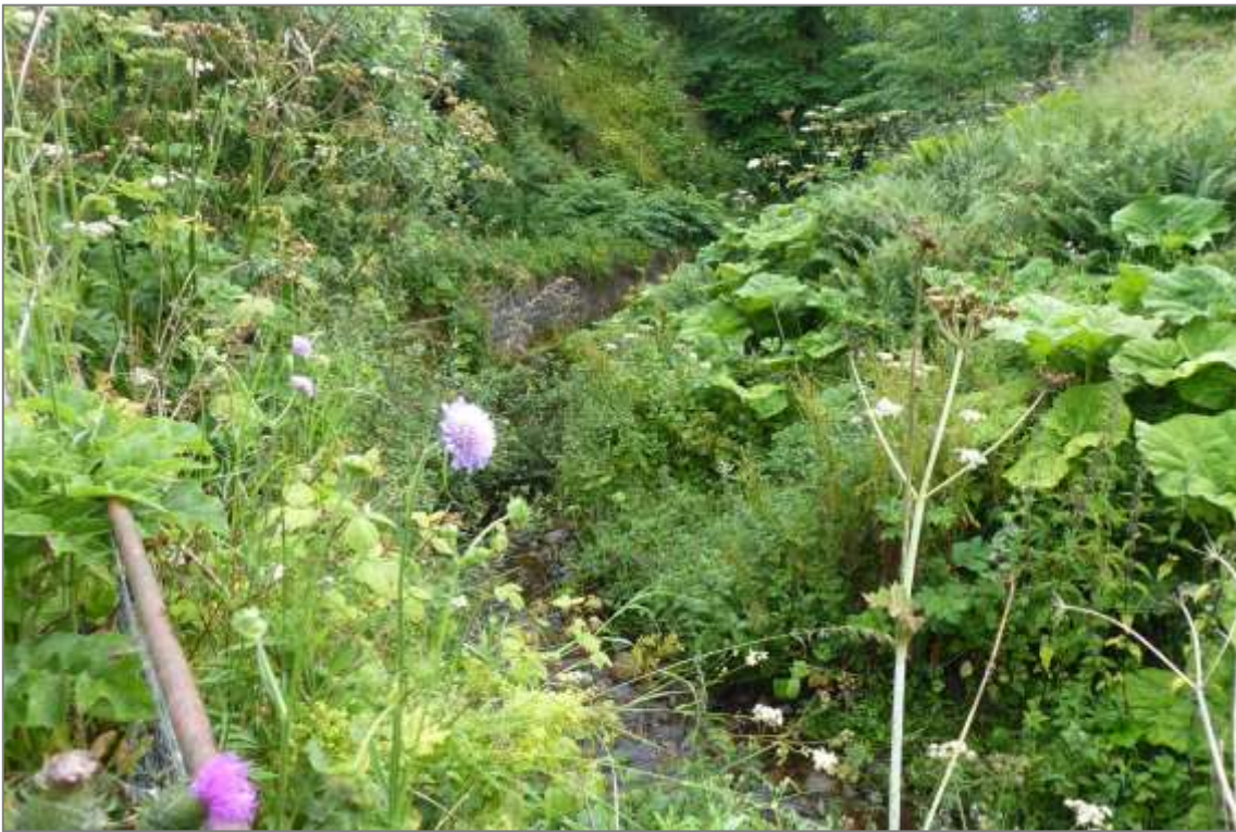
The Burn of Benholm at the high of summer with vegetation almost completely obscuring the burn retaining wall; inspection and grounds maintenance required during winter session to form repair strategy.
