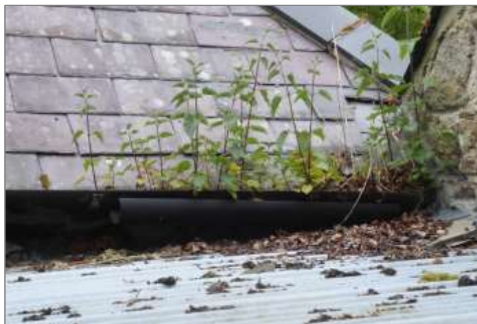
Detail of the defective junction of the kitchen extension roof and the shop wall; the gutter is blocked and a temporary section of gutter appears to have been placed below the existing gutter.
