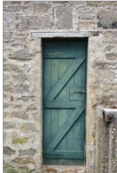
Meal mill: decayed timber lintol over later internal doorway now forming part of the external wall of the extension
