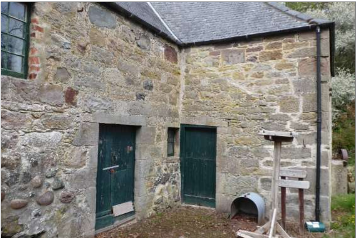
Mill of Benholm, meal mill south elevation meeting the L-plan extension. Note on the lowered left, the older field stone rubble wall is interrupted by the insertion of the doorway in 1817. The upper south elevation is of a later different masonry build as is the west facing elevation of the extension, where its earlier single storey pitched roof line is still evident. Above that a later build again as the extension was heightened and lengthened.
