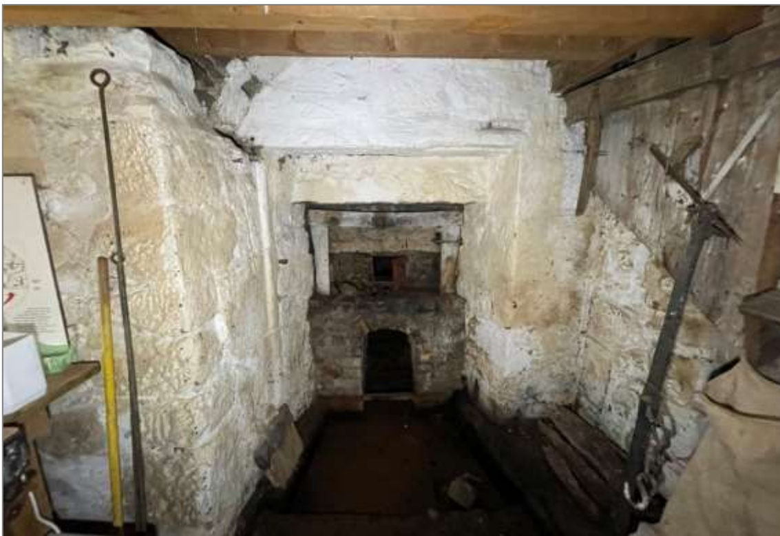
Mill of Benholm, meal mill kiln firebox on the lower floor. Note the deep wall construction part of which is thought to be an earlier doorway. Staining (damp) on paintwork around kiln opening.
