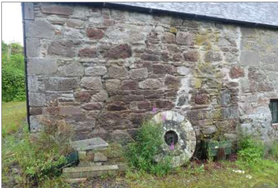
Meal mill: kiln south elevation showing poorly patched diagonal cracks, possibly as a result of movement
