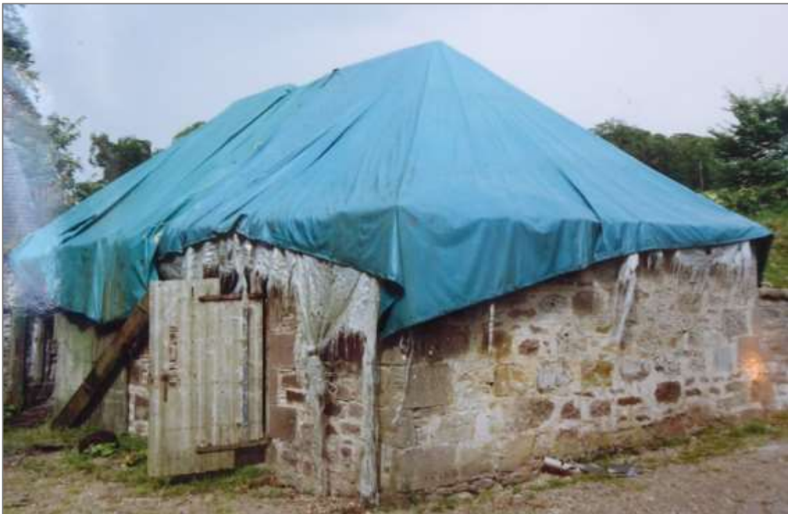
Mill of Benholm, byre prior to adaptation, note the original cast iron door hinges which were retained (HES file image, c.1992).
