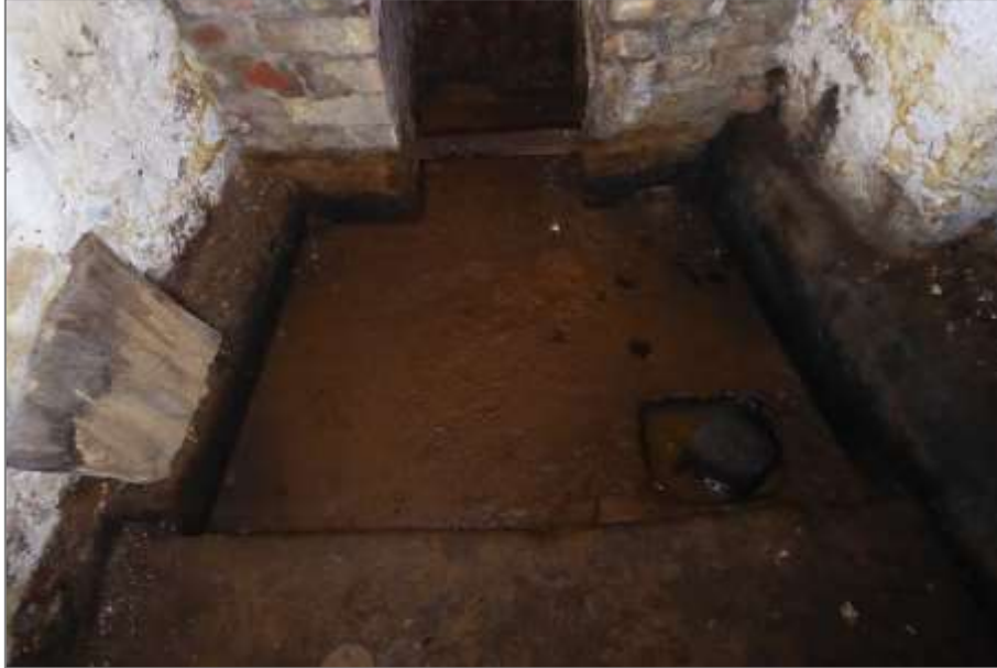
Ash pit in front of the kiln fire box showing silt build up from repeated water ingress and water sitting in a lowered area, possibly a blocked drain.
