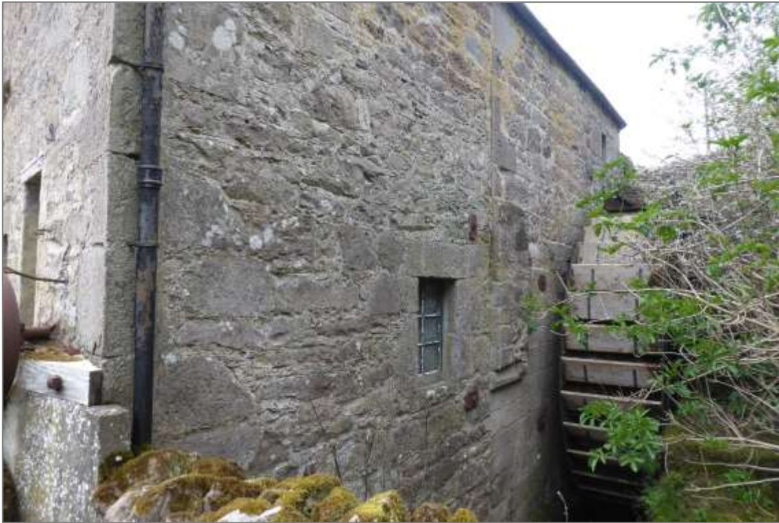
Mill of Benholm, meal mill east elevation showing a variety of masonry construction including smooth ashlar behind the lower waterwheel, and protruding masonry.
