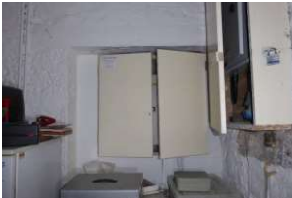
Original side entrance doorway within the byre now infilled with painted timber lintel.
