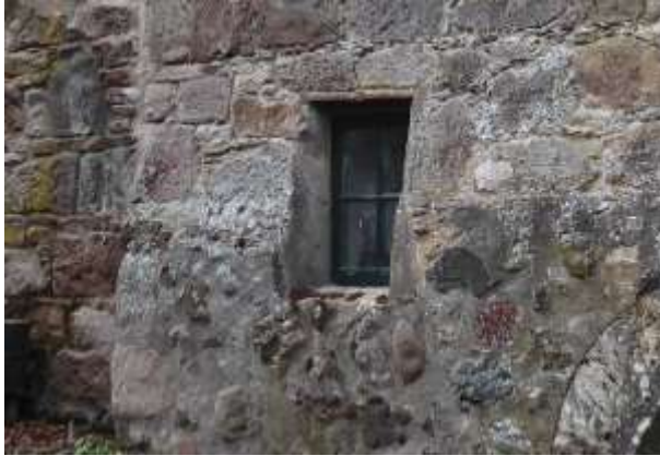
Small 4-pane fixed glass window with lintel formed by iron bar suggesting the window is a later alteration.
