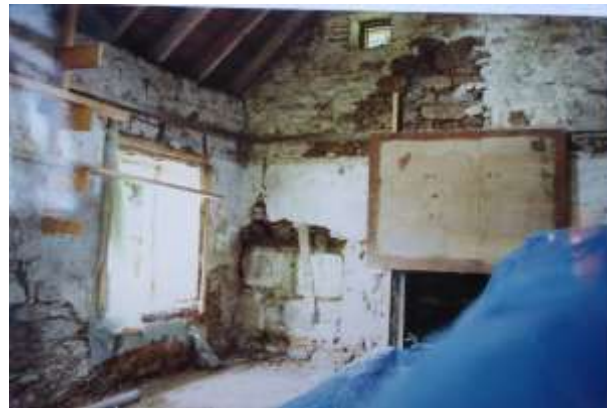
An image during adaptation shows the interior stripped back and the attic floor removed. The interior shows evidence of a possibly lower roof line showing as an unpainted part of the gable (HES file image, c. 1992).
