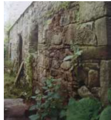
Photograph prior to the adaptation suggests the rear door was present prior to that, possibly roughly formed when the building was used as a byre (HES file image, c.1992)
