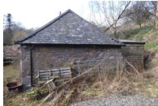
General view of the side (east) elevation where cement mortar pointing from its adaptation is visible.
