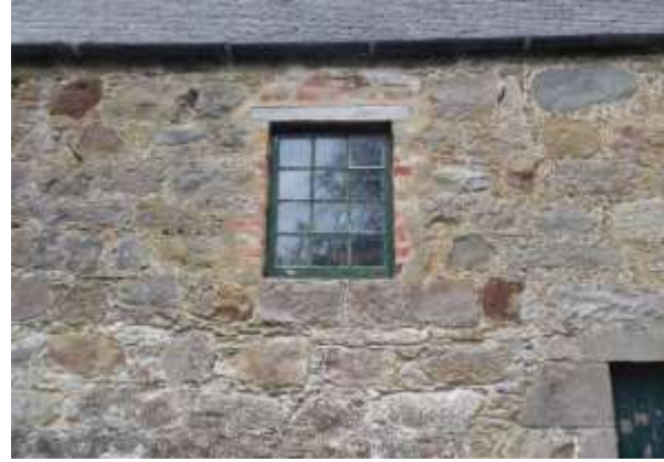
The upper section of the south elevation is coursed rubble of generally pale pink-grey sandstone using roughly squared blocks with the same small pinning stone detail found on the north elevation. Large 12-pane fixed glass window with timber lintels and brick jambs, again indicating this is a later alteration.
