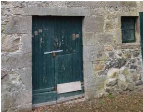
Principal entrance on the south elevation with double vertically boarded doors; the lintel is inscribed "William Davidson 1817" with inscribed initials on the adjoining stones. Small 4-pane fixed glass window to RHS with stone lintel.
