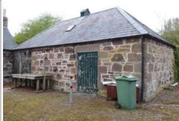
General view of showing the large boarded door. Iron handing bracket on LHS of door.
