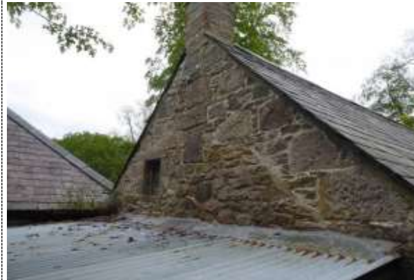
The height of the earlier gable may have been reduced whilst rebuilding to accommodate the large wallhead stones now evident.
