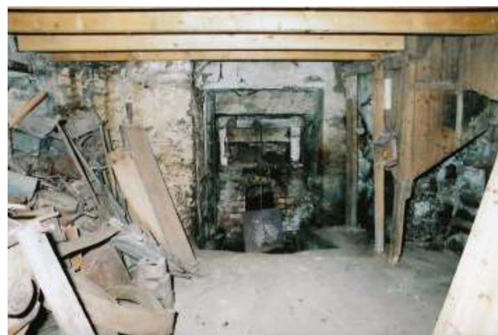
Similar view taken by WE Ltd during the restoration works. The kiln fire pit is visible with the Kiln Chute to the right. Note the new timber floor joists above.
