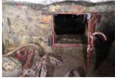
Kiln fire damper .
