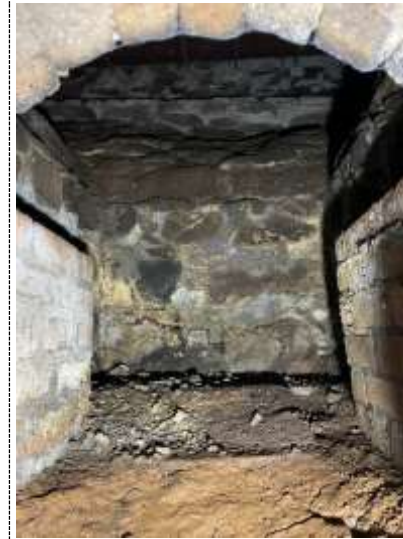
View into the fire pit showing the built up construction forming the funnel shape below the wire mesh floor above.
