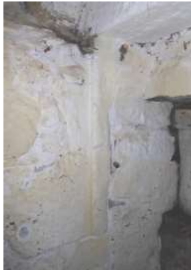
Detail of wall forming the kiln opening on the south side – evidence of dressed stone opening.
