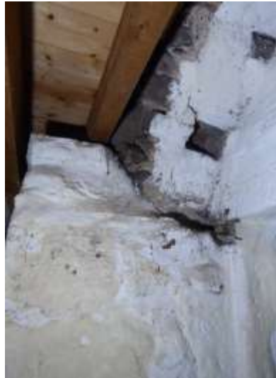
Detail of wall above forming the kiln opening on the south side – possible joist / timber rafter pockets.
