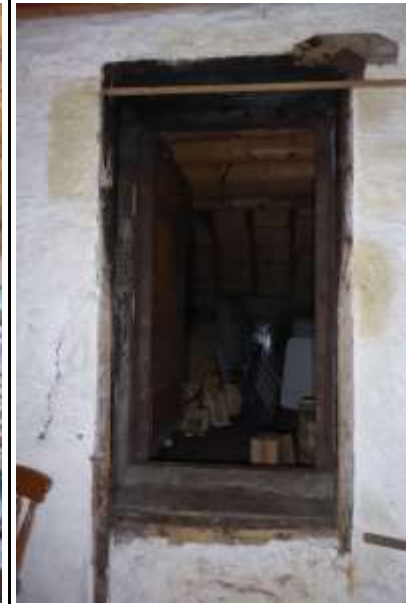
(Above) view from milling room. Large door opening with stone kerb/cill, timber frame flush to internal mill wall and timber lintels (charred). Iron door and door frame set back in line with internal wall of kiln. Wedge wire mesh floor, raised above FFL at c. 500mm. Raised concrete kerb around kiln floor with metal trim. Opening in west external wall with timber boarded hinged cover.
