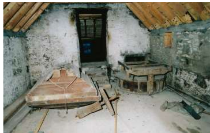
Similar view taken by WE Ltd during the restoration works, c.1991. Note dismantled milling items, repointing of walls with inappropriate cement and new timber rafters.
