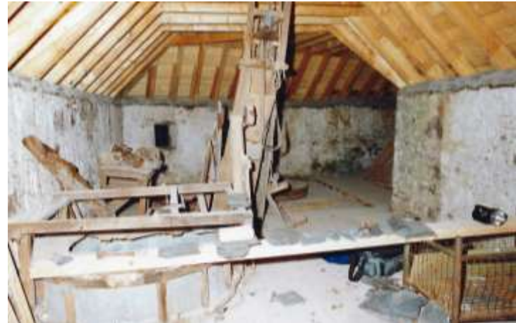
Similar view taken by WE Ltd during the restoration works, c 1991. Bag Hoist and Bucket Elevator prior to repair in the foreground, milling stone casing removed.
