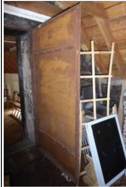
View of the external metal door face from inside the kiln.
