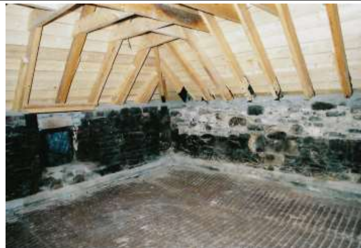
WE Ltd image during the restoration works, c.1991 of the kiln interior. Note repointing/rebuilding of walls with inappropriate cement and new timber roof construction. This floor probably dating to 1971 when a fire destroyed the kiln roof.
