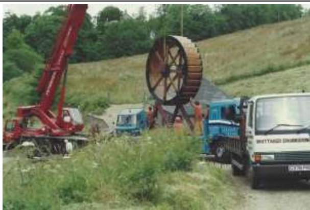
WE Ltd delivering the new waterwheel for installation in April 1992 (WE Ltd image).
