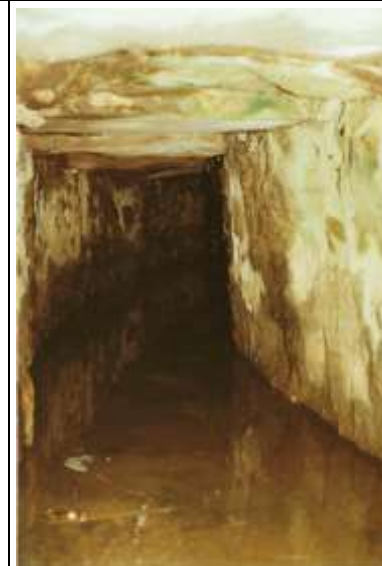
View within the tailrace during the restoration works c. 1991. (WE Ltd image).
